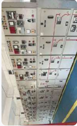
11kV/33kV VCB Panel (Vacuum Circuit Breaker)
