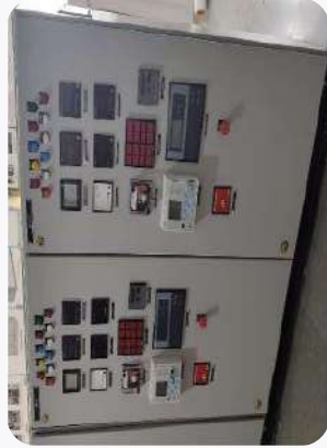
Control & Relay Panels (CRP) up to 33kV
