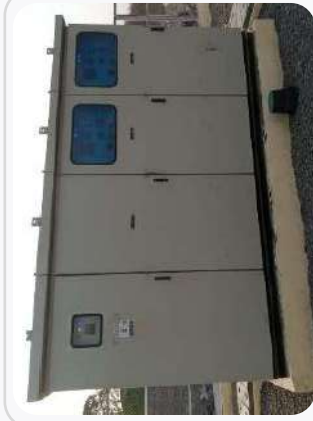
33kV RMG Panel
