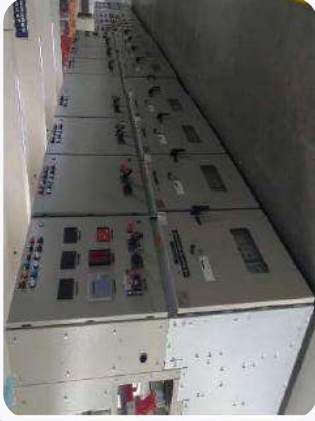
11kV DG Synchronizing & Load Sharing Panels
