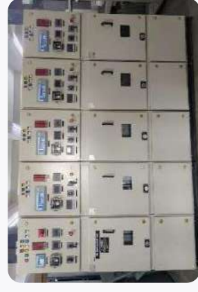
11kV Vacuum Contactor Panel
