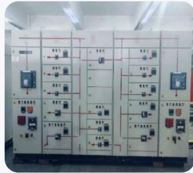
Motor Control Centres (MCC) Panel
