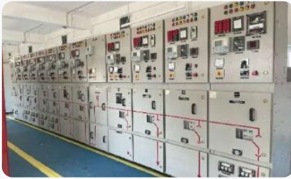
11kV/33kV VCB Panel (Vacuum Circuit Breaker)
