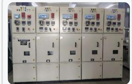
11kV Vacuum Contactor Panel
