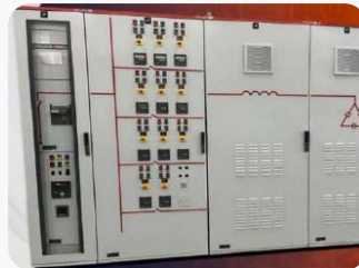
Automatic Power Factor Correction (APFC) Panel
