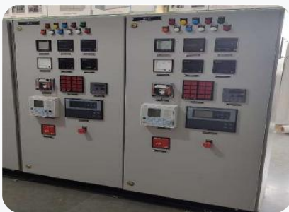
Control & Relay Panels (CRP) up to 33kV
