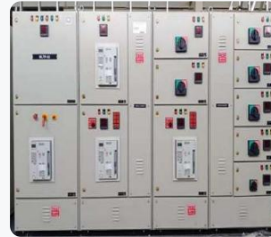
Intelligent Motor Control Centre (IMCC) Panel
