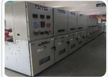
11kV DG Synchronizing & Load Sharing Panels
