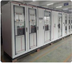
Power Control Centres (PCC) Panels
