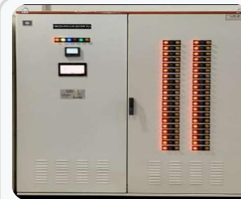
Power Distribution Unit (PDU)
