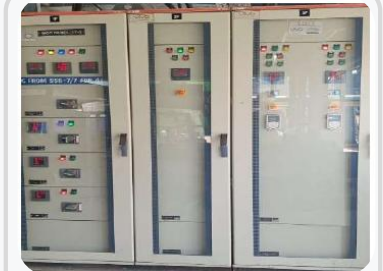
Variable Frequency Drive (VFD) Panel
