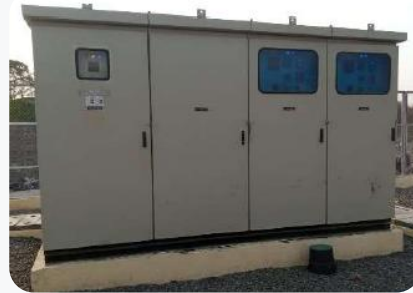
33kV RMG Panel
