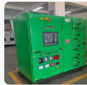
DG Synchronizing & Load Sharing Panels
